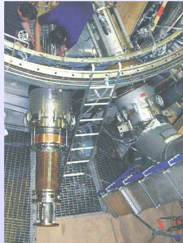
70 kA HTS CL installed in TOSKA
