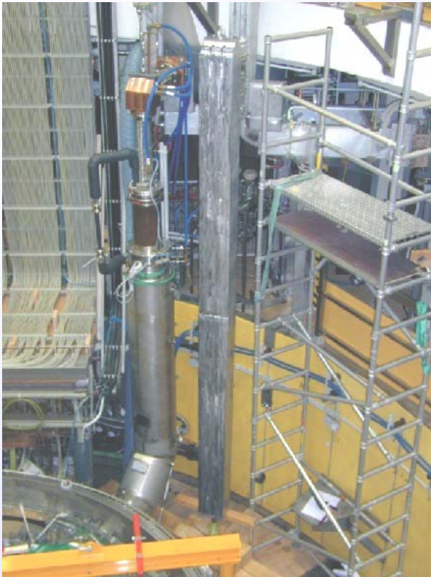
Conventional(LTS) 80 kA CL and Aluminium bus bar installed in TOSKA
